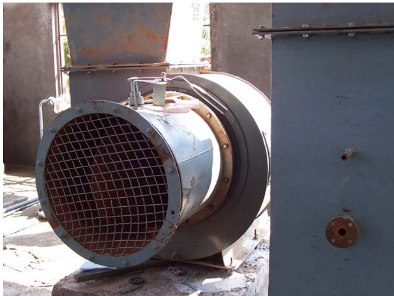
Photo 1: One more installation with flap damper right at the fan inlet.
